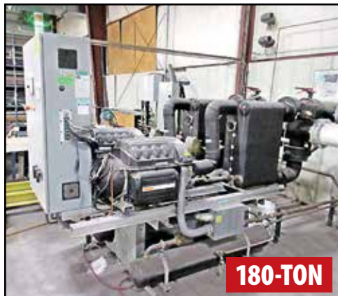
2012 THERMAL CARE TRC 180 CHILLER
