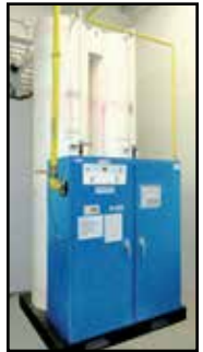
ON-SITE GAS SYSTEM NITROGEN GENERATOR
