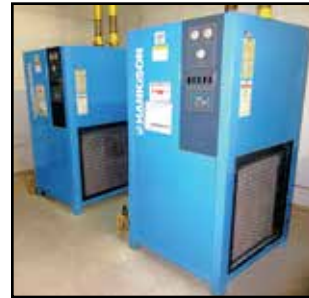
(2) HANKISON AIR DRYERS
