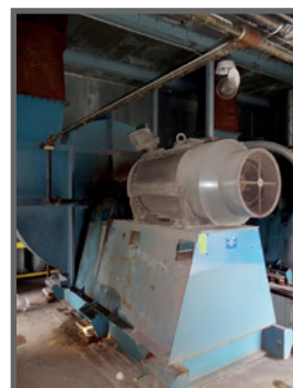
500 HP TECO WESTINGHOUSE BCN-SW BLOWER
