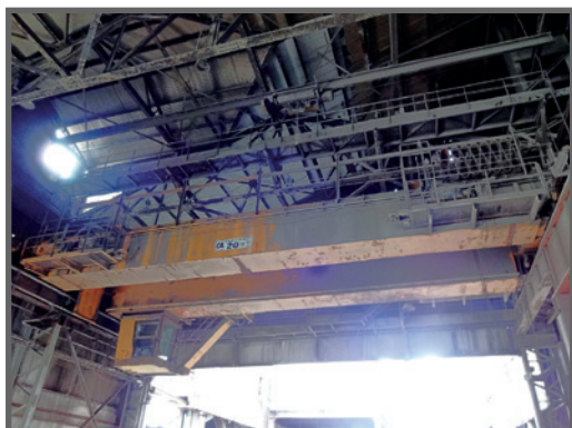
20 TON ALLIANCE BRIDGE CRANE
