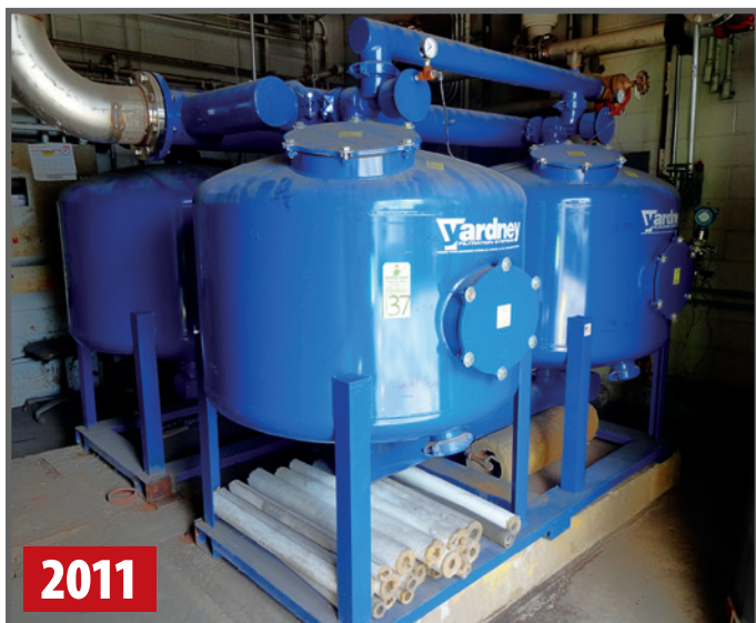
2011 YARDNEY RCW4824-4AS COOLING TOWER SAND MEDIA FILTER
