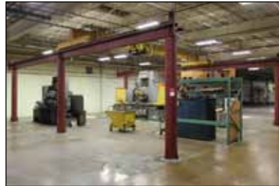
5 Ton OMI Bridge Crane with Electric Hoist
