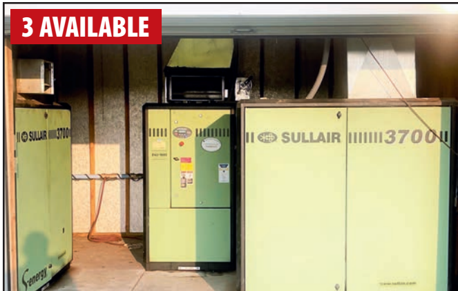
VIEW OF SULLAIR 55 HP AIR COMPRESSORS
