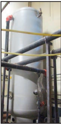
(1 OF 2) AIR RECEIVER TANKS
