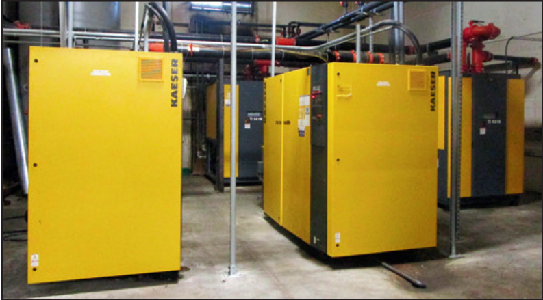
VIEW OF KAESER AIR COMPRESSORS AND DRYERS
