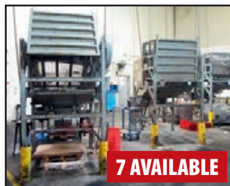
(3) BIN DUMP/SORT STATIONS
