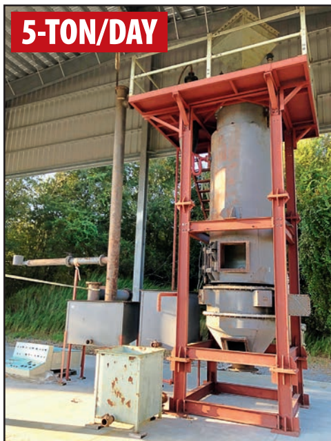
RADHE BIOMASS/COAL GASIFIER SYSTEM
