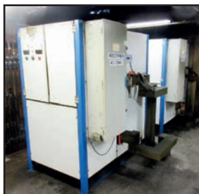
(2) NORTH AMERICAN RECTIFIER 6PF-F 12,000 AMP RECTIFIERS
