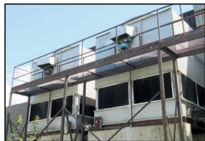
(2) EVAPCO COOLING TOWERS
