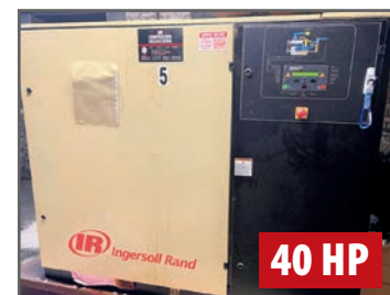
INGERSOLL RAND AIR COMPRESSOR
