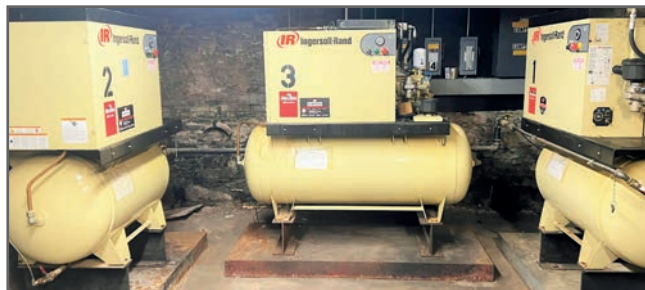
(3) INGERSOLL RAND 15 HP AIR COMPRESSORS
