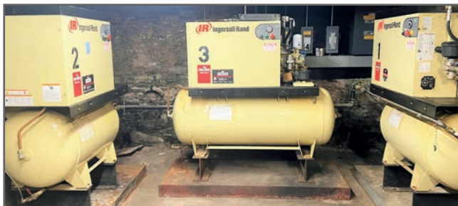
(3) INGERSOLL RAND 15 HP AIR COMPRESSORS
