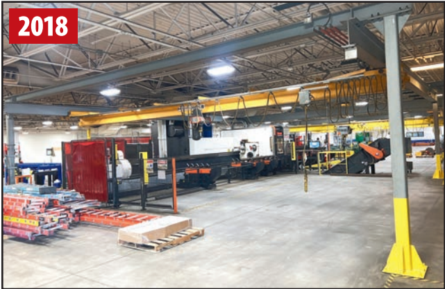
HS 1.5-TON CRANE SYSTEM
