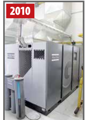
(2) 223 HP ATLAS COPCO GA160FF AIR COMPRESSORS
