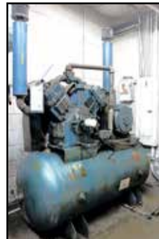
DUAL PISTON AIR COMPRESSOR 25 HP W/200-GALLON AIR TANK
