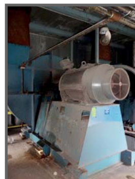
500 HP TECO WESTINGHOUSE BCN-SW BLOWER
