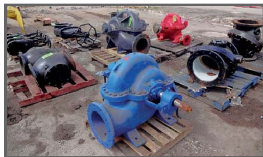
VIEW OF PUMPS AND VALVES
