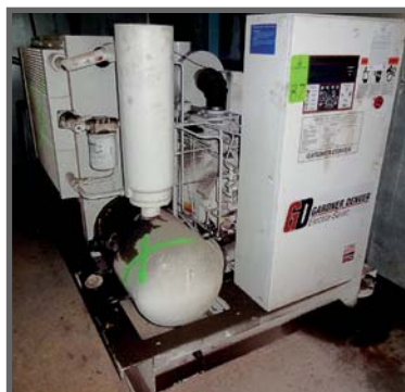
100 HP GARDNER DENVER EAP99J AIR COMPRESSOR
