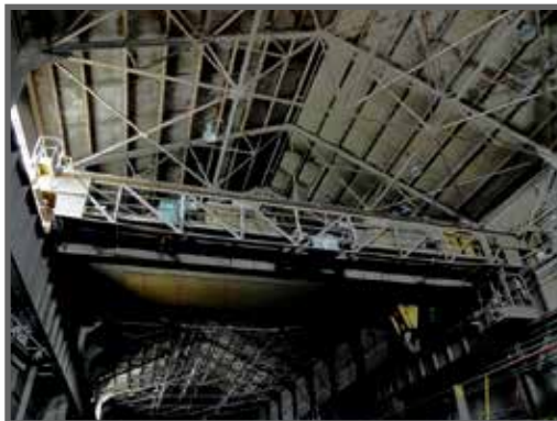
125 TON MORGAN BRIDGE CRANE
