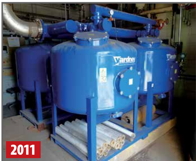
2011 YARDNEY RCW4824-4AS COOLING TOWER SAND MEDIA FILTER
