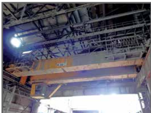
20 TON ALLIANCE BRIDGE CRANE
