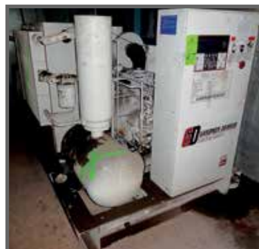
100 HP GARDNER DENVER EAP99J AIR COMPRESSOR
