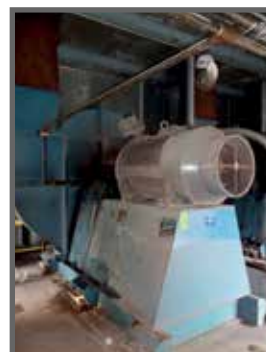
500 HP TECO WESTINGHOUSE BCN-SW BLOWER
