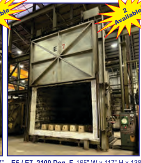
E5 / E7, 2100 Deg. F, 165" W x 117" H x 138" D, natural gas, 6 burners, fiber lined, Honeywell controls
