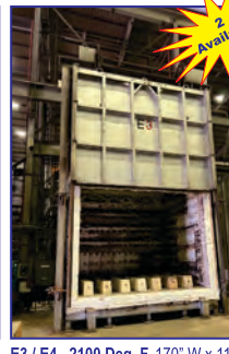
E3 / E4, 2100 Deg. F, 170" W x 117" H x 140" D, natural gas, 6 burners, fiber lined, Honeywell controls
