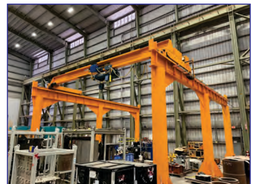
(above) 10 Ton Shaw Box Crane Free Standing System , 10 ton cap.,
