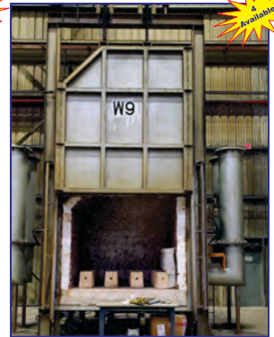
W9 / W10 / W11 / W12, 1850 Deg. F, 98" W x 68" H x 82" D, natural gas, 2 burners, fiber lined, Honeywell controls
