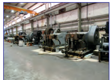
General Views of Press Pumps
