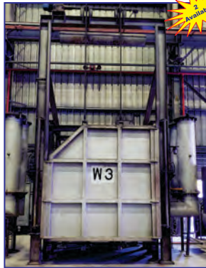
W3 / W4 , 1850 Deg. F, 96" W x 61" H x 86" D, natural gas, 2 burners, fiber lined, Honeywell controls
